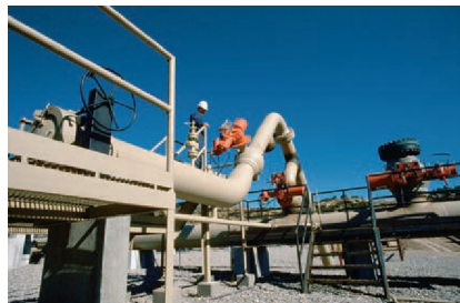
▲ Figure 10.15 A natural gas pipeline junction.
